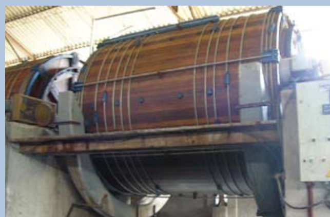
New equipment installed at the plant
